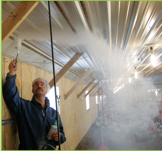
Shown here is the use of a smoke generator to evaluate air flow; which in this case is poor. You can see cold air dropping directly onto the floor. Proper minimum ventilation allows for mixing of cold air with warm moist air.
